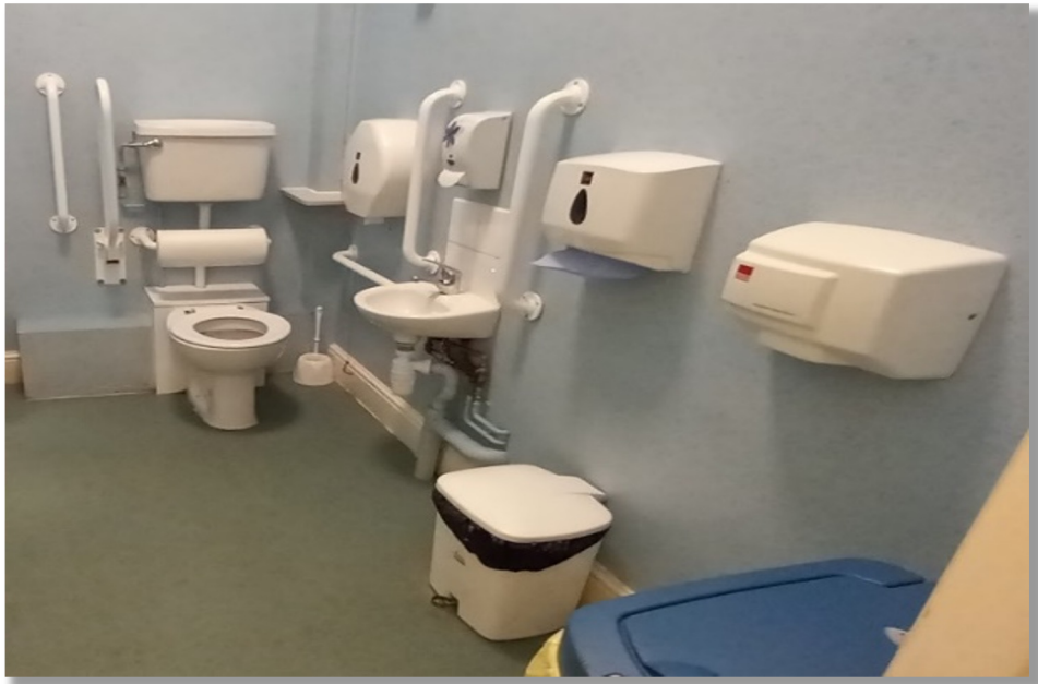
The accessible toilet on the Ground Floor with white vertical and horizontal grab rails, toilet accessories and toilet
